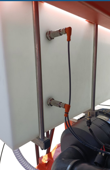
Water level switches
