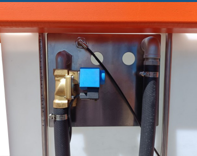
Solenoid valve for water supply
