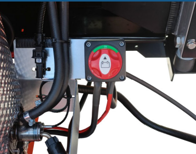
Main battery switch
